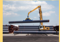
Vacuum System for Pipe Loading
